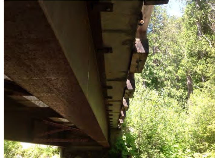
deck clips - 1 missing downstream
