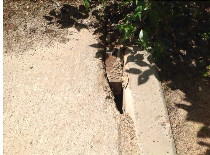
left approach 1st panel damage
